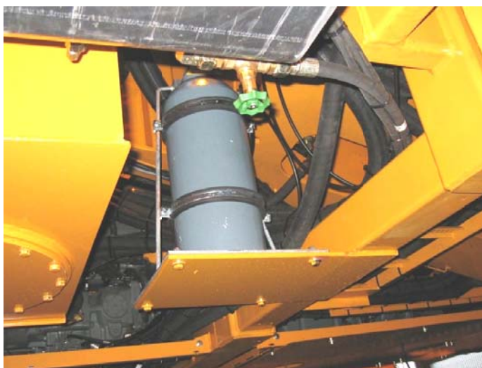
10 kg powder extinguisher fixed on a galvanised massive holder outside the excavator.
